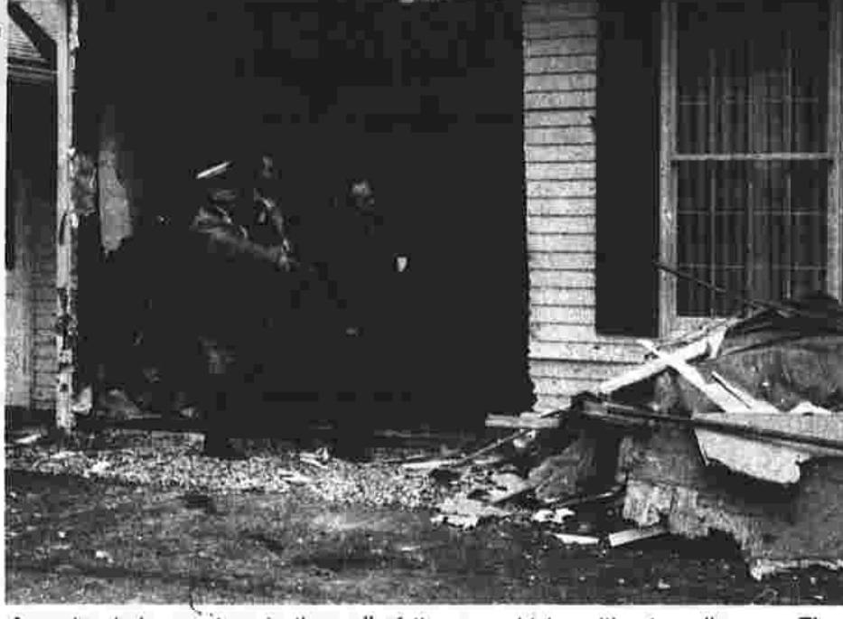
A gaping hole was torn in the wall of the Faith Baptist Church, 52 Lake St., Manchester, when a van veered off the road. The driver, Henry Owens, 17, of 19 Redbird Lane, Glastonbury was charged with reckless driving and operating a motor vehicle without a license.
